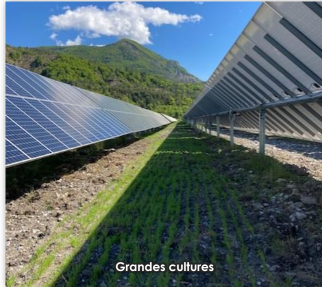
Trackers photovoltaïques (espace test) – Curbans (04)
